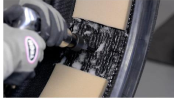
Use Carbide Cutter to Remove Damage
