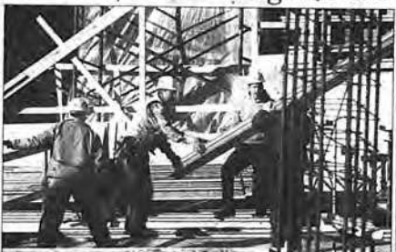
Construction is under way on the Millennium Center condominiums on Ontario Street. Spending on construction rose just 0.2 percent in December, well below analysts' expectations.
