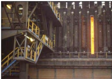
Coke Ovens at smokeless fuel plant Abercrombie - (Source : Wikipedia )
