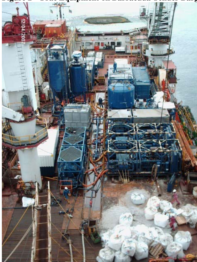
Figure 2 – Frac Equipment on Barracuda Tender Barge
