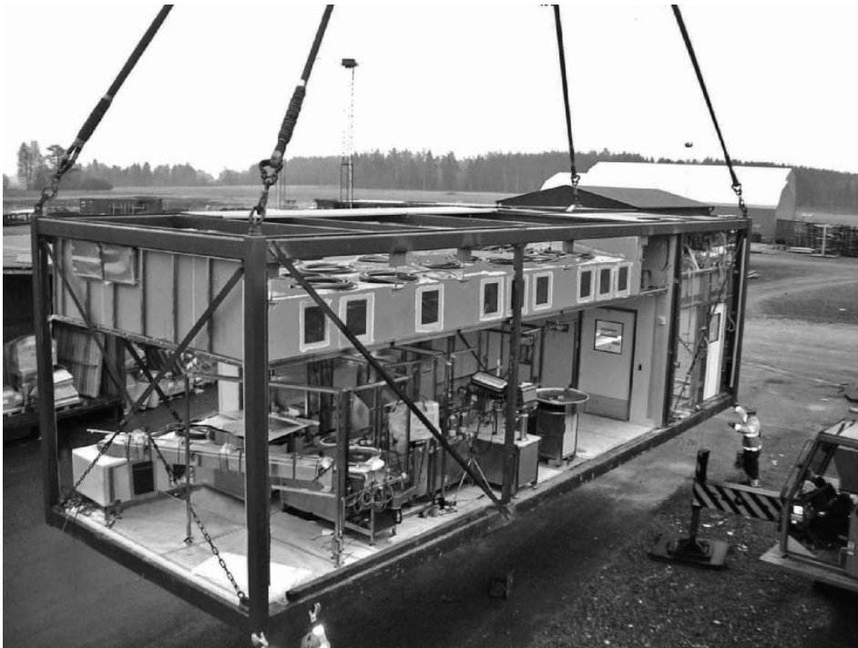
Figure 14-5 Example of a modular unit for a sterile manufacturing facility. Source: Courtesy of Pharmadule, Inc.
