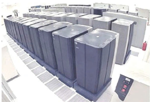
Fig. 1. Physical organization of a data center.
