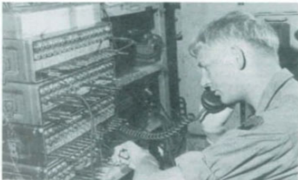
SB-22 SWITCHBOARD aboard the Benewah.
