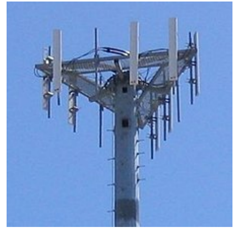
A multi-directional, cellular network antenna array ("cell tower")
