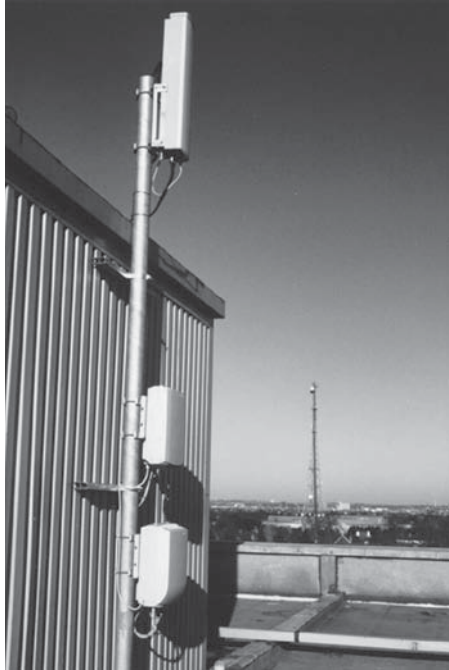
Figure 4.28 Roof-top mounted sector site consisting of antenna unit with integrated amplifiers, micro base station, and battery backup unit (Courtesy of Ericsson)
