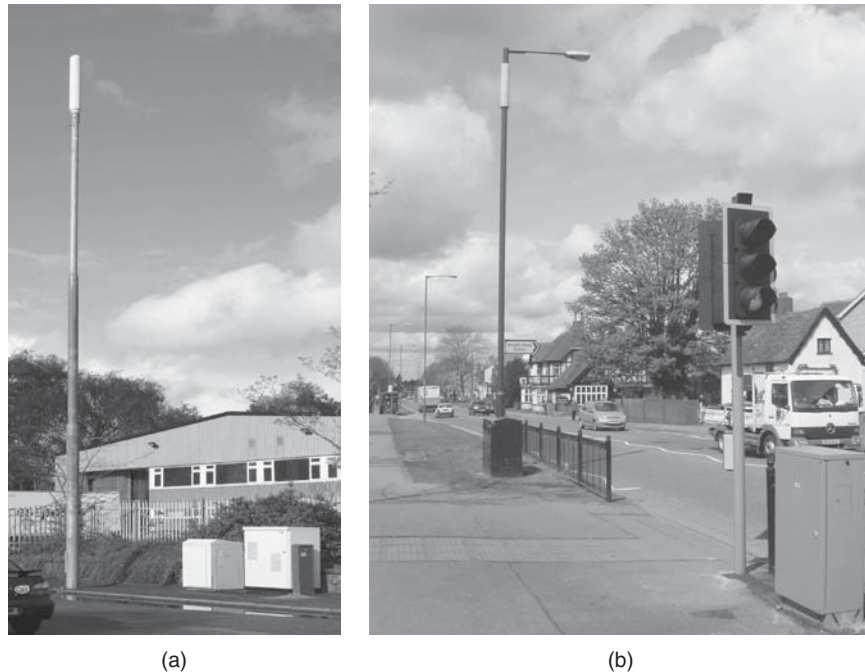
Figure 2.21 These base stations quickly become part of the street scene and are hardly noticed by the average passerby. (Photos by the author)
