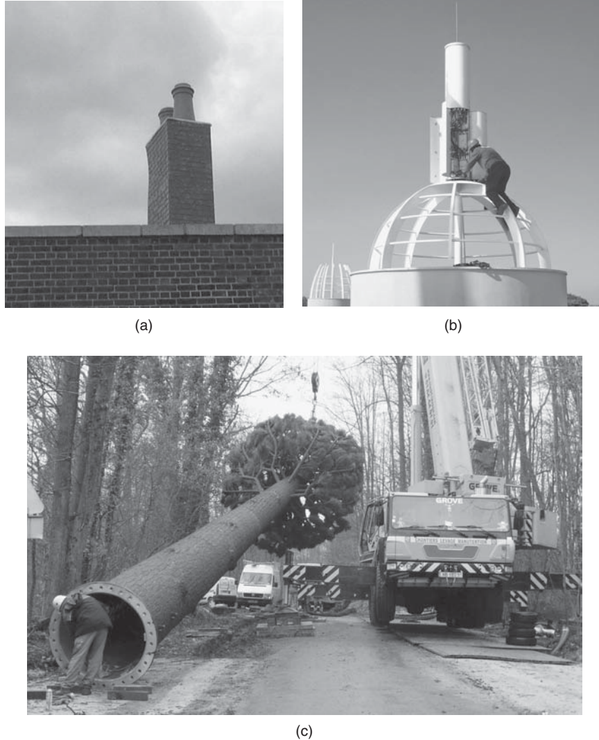
Figure 2.22 Disguised base station antenna solutions: (a) A grp structure surrounding the antenna (Photo courtesy of Jaybeam Wireless); (b) an integrated three-sector BS antenna with TMAs presented as an architectural feature (Photo courtesy of Powerwave, Inc.); and (c) a BS disguised as a tree being lifted into position (Photo courtesy of Kitting Telecom)
