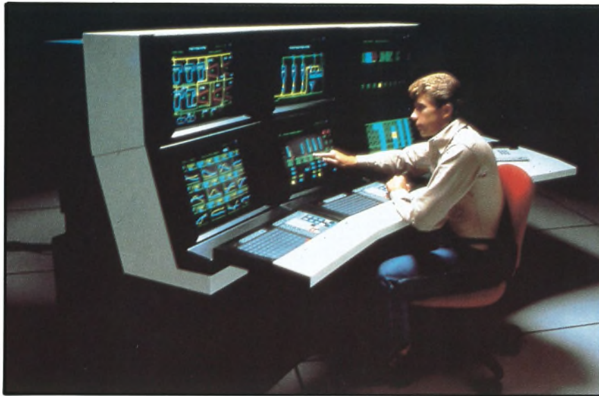
Figure 7. An example of a process control system: operators use touch-screens to monitor processes and modify parameters if needed.
