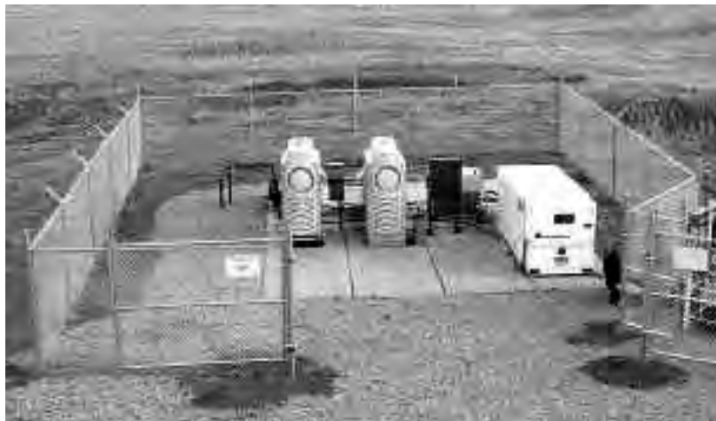
FIGURE 39.15 Aerial view of the PowerBlock® module with two microturbines near the Denver International Airport. (Source: From Reference 22.)
