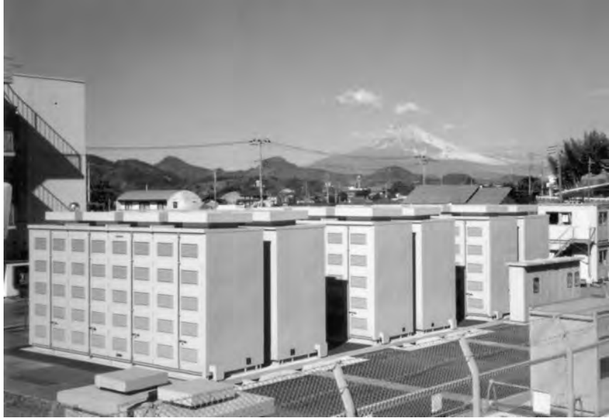
FIGURE 40.16 A photograph a 6 MW/ 48 MWh NGK sodium/sulfur battery system that is operating in a load-leveling mode at Ohito, Japan. This battery is one of the two largest sodium/sulfur batteries ever built and has been operating since early 1998 (Courtesy of Tokyo Electric Power Company and NGK Insulators, Ltd.).
