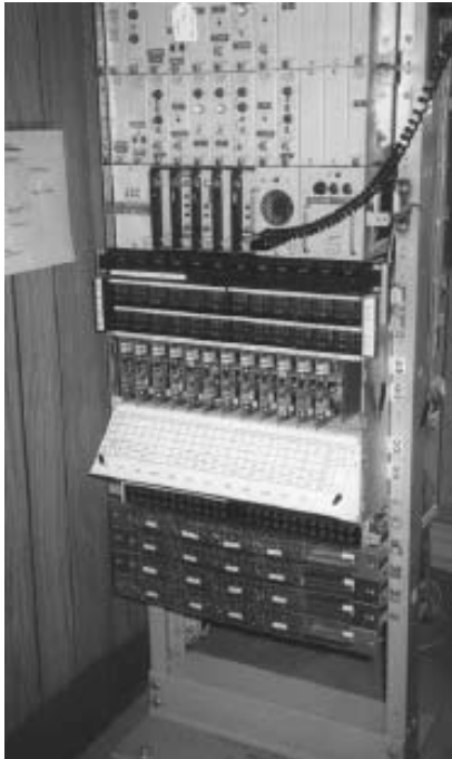
Figure 3: A 12-channel frequency division multiplexing (FDM) equipment bank used in an analog microwave system for telephony. Copyright © 2002 Dave Whitmore. Reprinted by permission.
