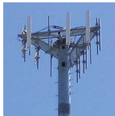
A multi-directional, cellular network antenna array ("cell tower")
