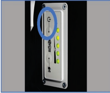
Figure 11, UPS Control Panel, On/Off Button circled
