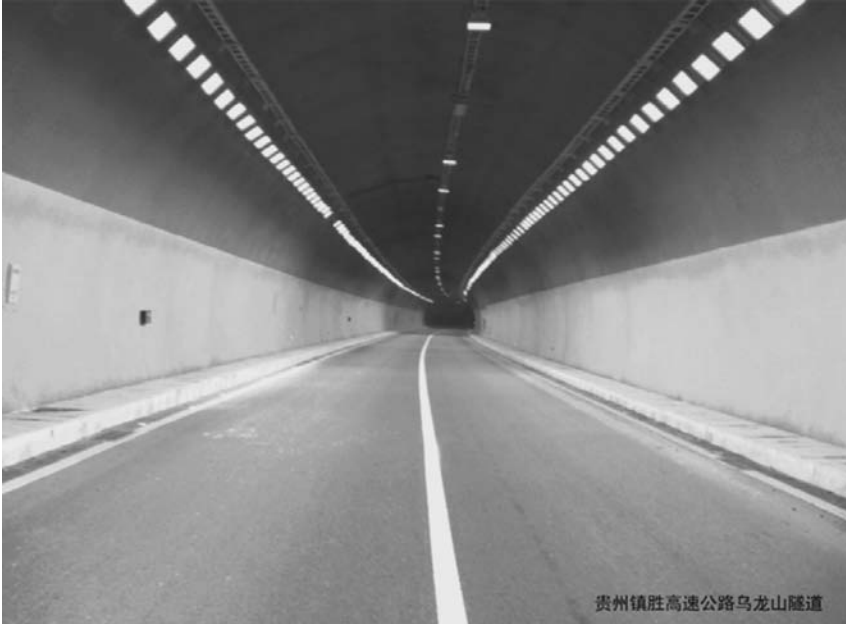
Figure 1.3 LED tunnel lighting in Guizhou Province, China. (Reproduced with permission from www.gd-realfaith.com , Guangdong Real Faith Enterprises Group Co., Ltd., accessed April 12, 2011.)
