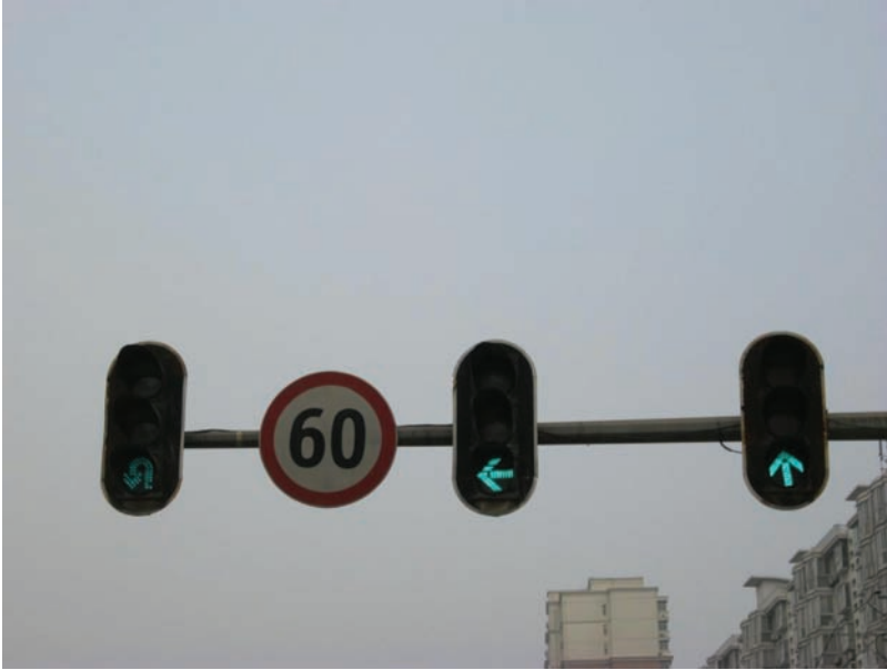
Figure 6.97 LED traffic signal lights. (Color version of this figure is available online.)
