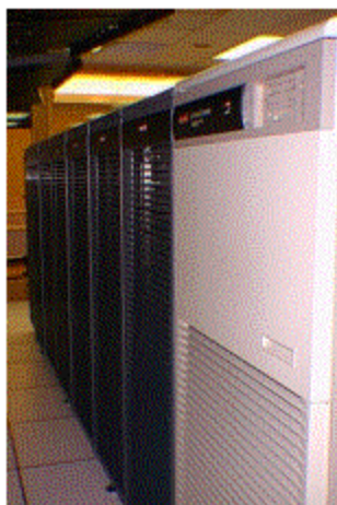
Figure 1. The TerraServer hardware
