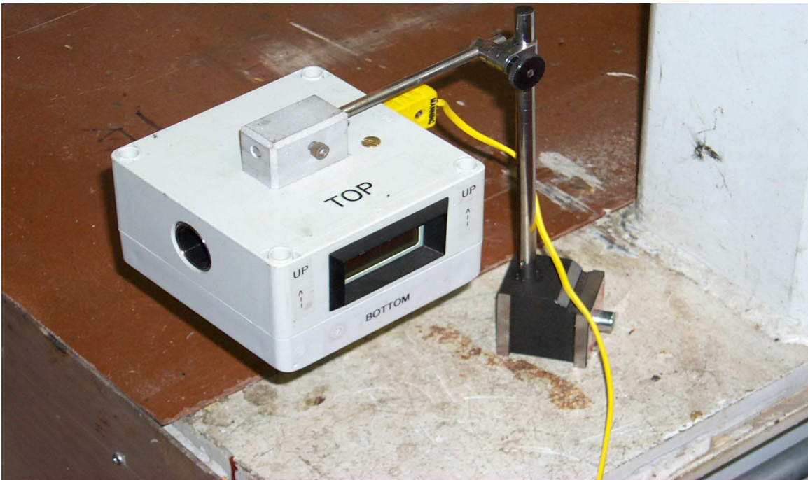
INFRARED SENSORS USED FOR NON-INTRUSIVE TEMPERATURE MONITORING - USED FOR HYDRO GENERATOR POLE PIECE CURING PROCESS AFTER RE-INSULATION
