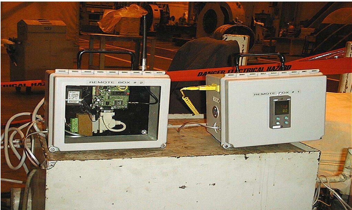
RADIO MODEM BEING USED DURING INITIAL ADM TESTING
