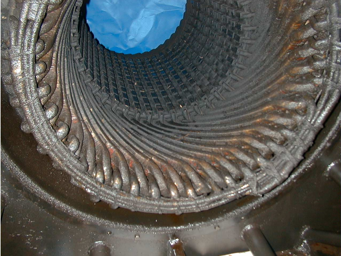
PHOTO SHOWING THE DIRT/OIL ON THE STATOR WINDING (BEFORE CLEANING)
