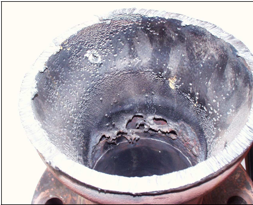
Figure 11. Plant C - Heater Drain Line –FAC Failure of Expander
