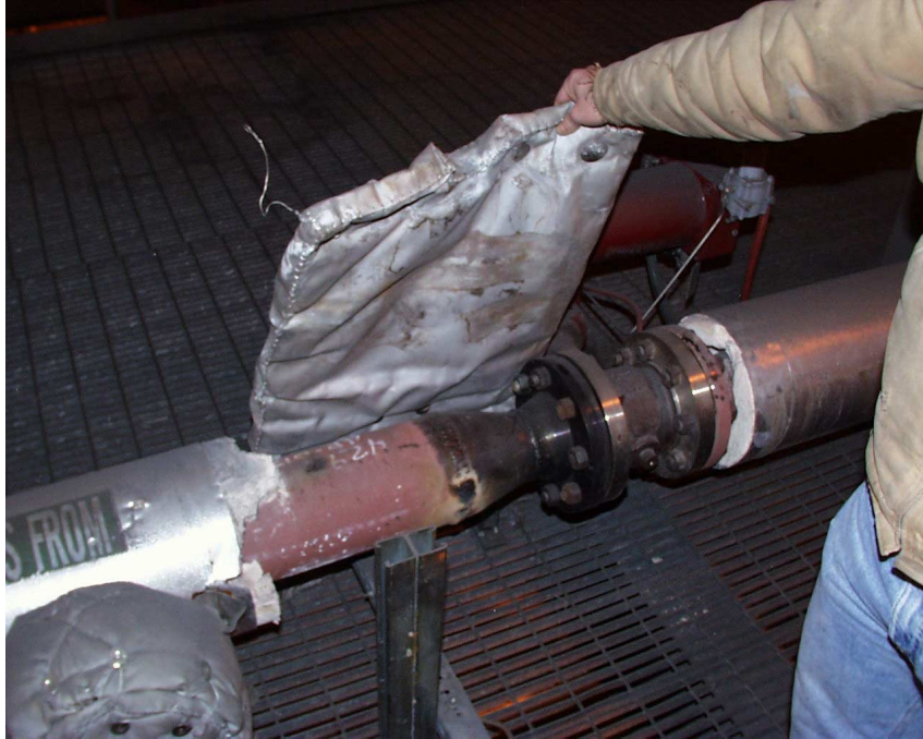
Figure 10. Plant C - Heater Drain Line –Repair of Expander Damaged by FAC
