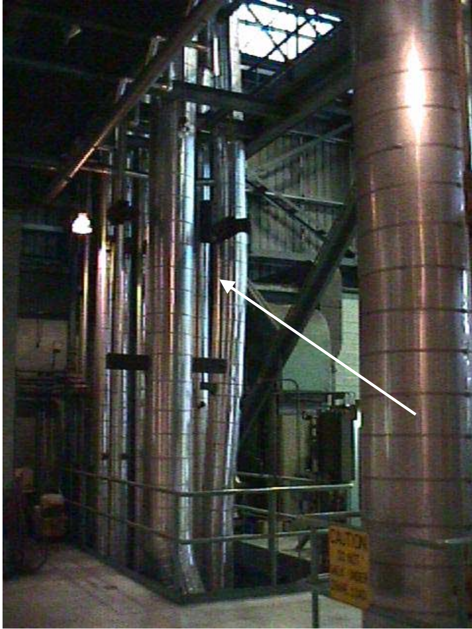
Figure 2. Plant A – 14 th Stage Extraction Line – Water Hammer Damage
