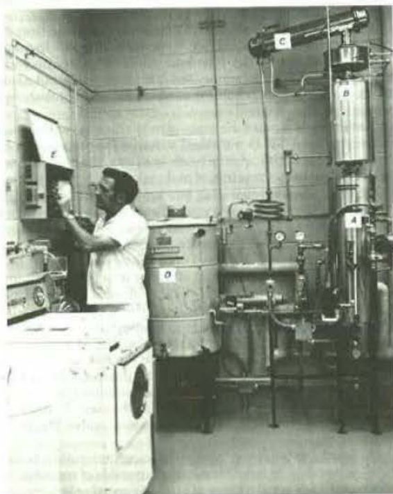
Fig. 84-2. High-purity still and sealed-water storage system. A: Evaporator; B: high-purity baffle unit; C: condenser; D: storage tank with ultraviolet lamp; E: control panel (courtesy, Ciba-Geigy).
