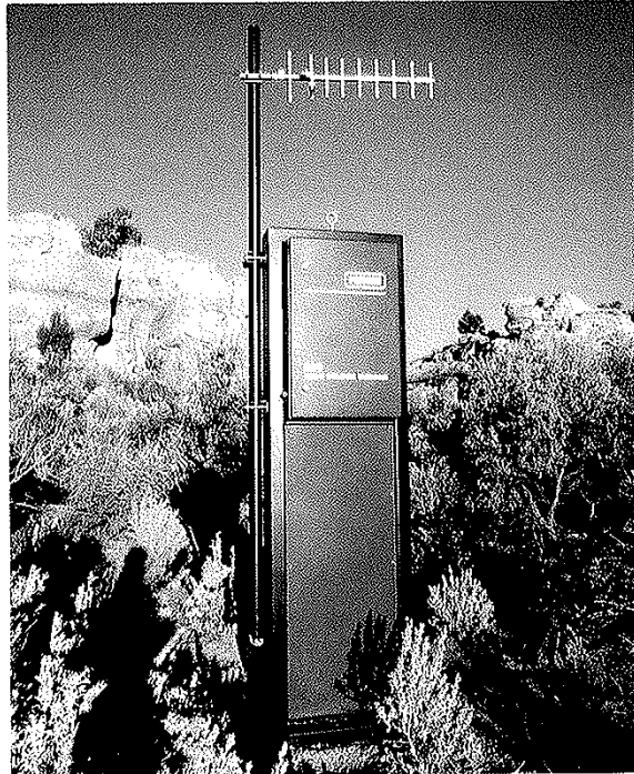
Remote units are available in tree-standing, weatherized enclosures for easy, low-cost installation.
