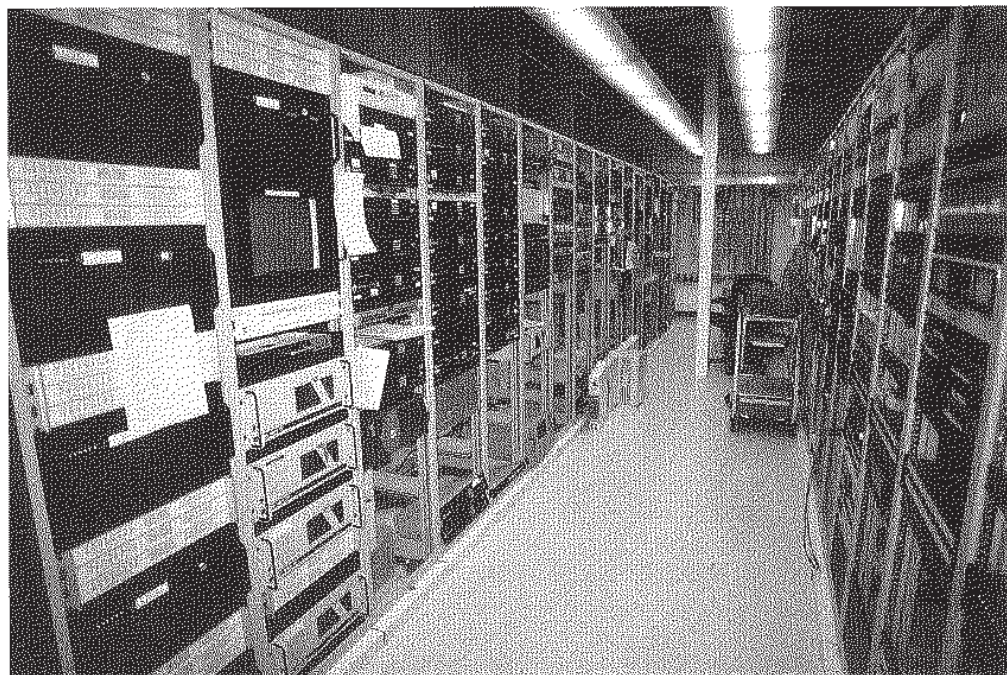
FIGURE 10.28 Rack rooms in cluster operation. Courtesy Clear Channel.
