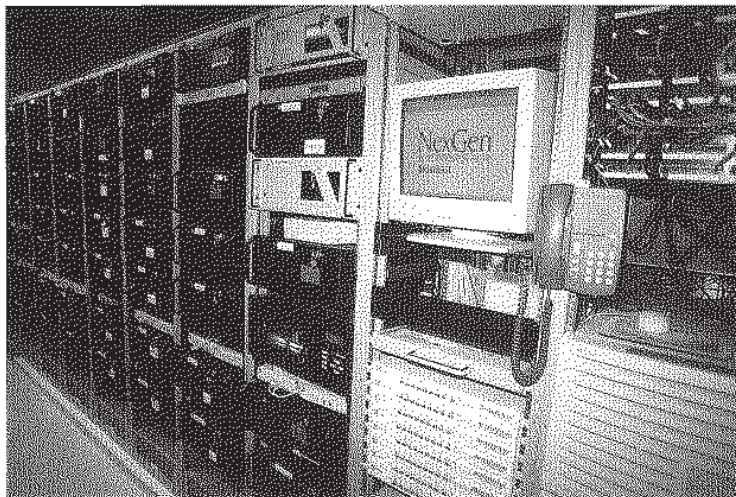
FIGURE 10.2 Station engineering operations in the digital age. Courtesy Clear Channel.
