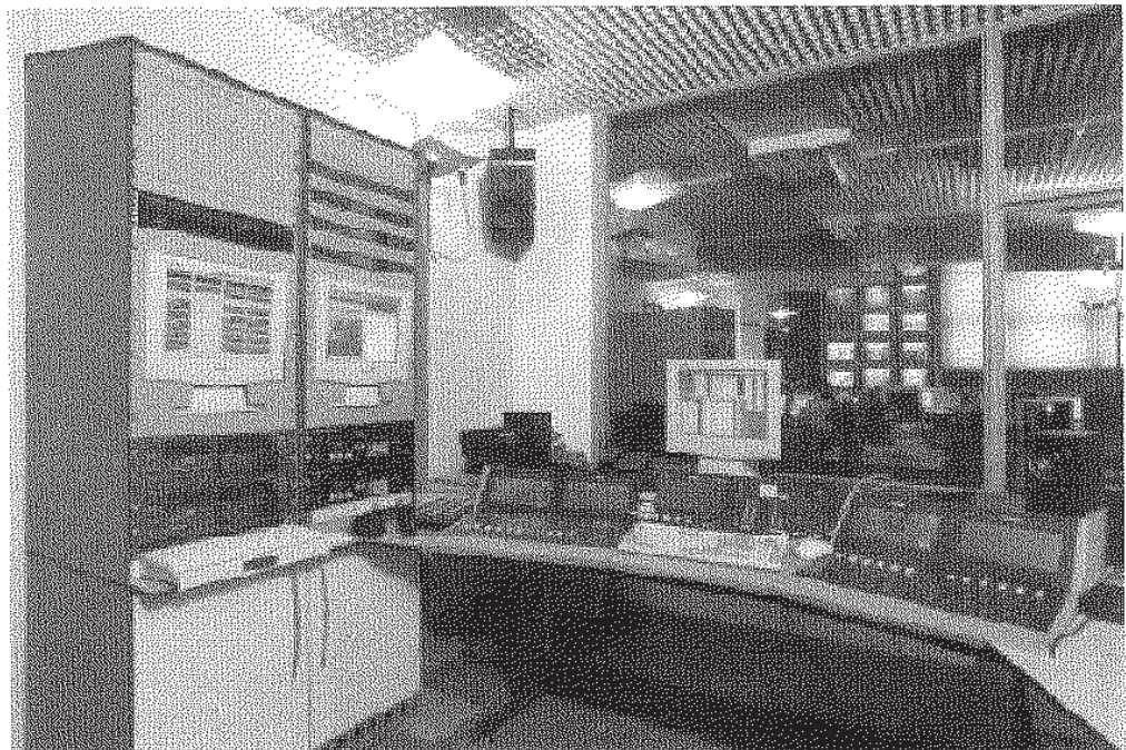
FIGURE 9.3 This cutting-edge digital studio is state of the art. Courtesy RTBF.
